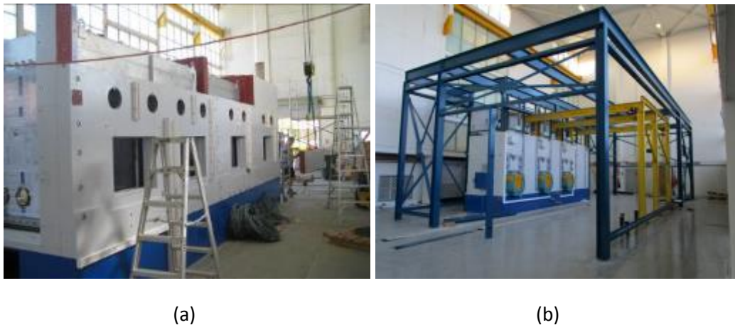
Figure 1 Assembly of the new ANSTO PIE hot cells as at (a) mid-October 2013 and (b) August 2014. The stainless steel confinement boxes are visible behind the lead shielding.
