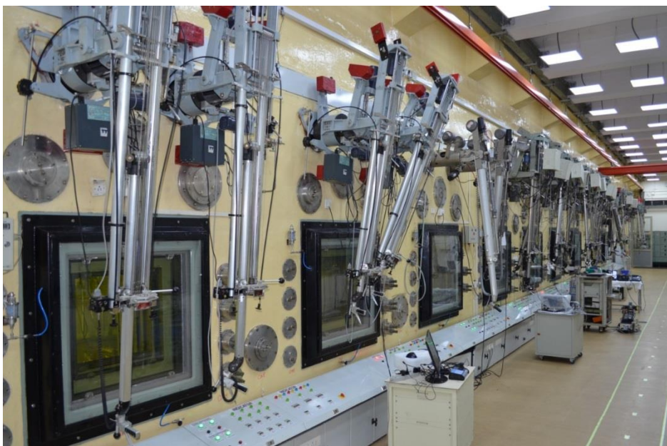
Figure 4: Operating area of the hot cells in the NHF showing the viewing windows and master slave Manipulators (MSMs)
