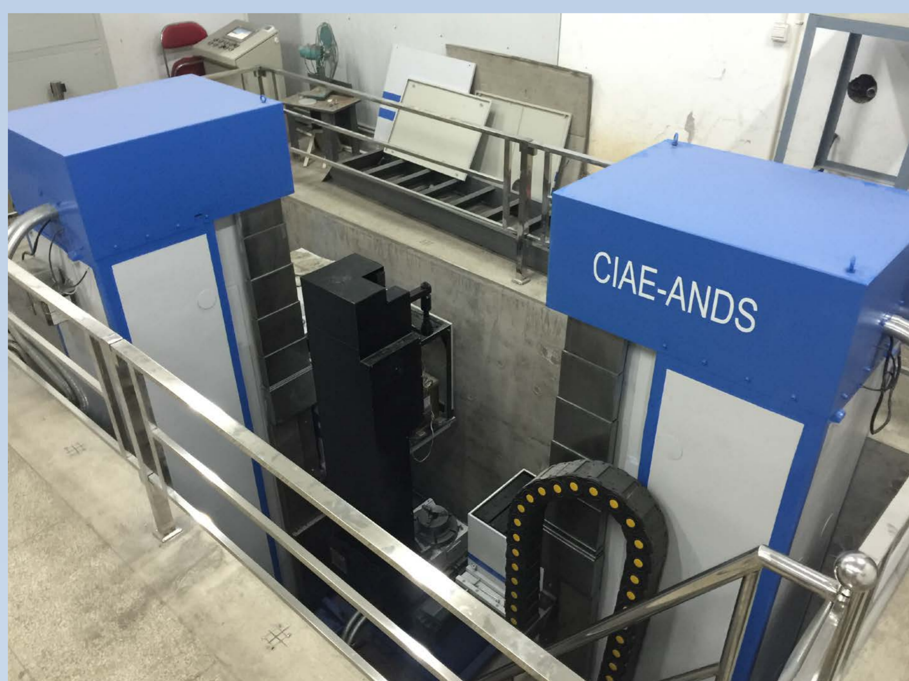
Figure 3. Facility for the detection of nuclear fuel assembly.
